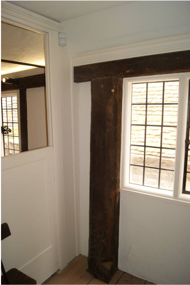
Figure 4 Sample location of OB02 Post in west wall. View to the west.
